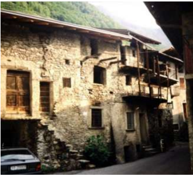
Fig. 10 Houses in Via Dessedo. Although re-roofed and in the process of reconstruction, the basic fabric probably dates from the 19 th century. Note particularly the balconies. Image courtesy of Alan
